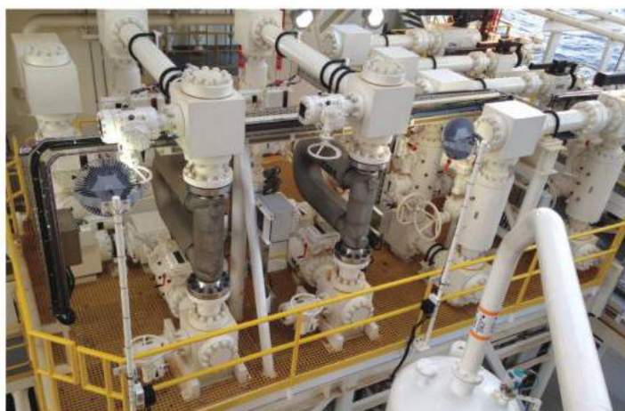
Rig owned MPD choke and meter manifolds. Complete with dual 3in and 6in chokes and dual 8in Coriolis meters. Photos from SafeKick.
